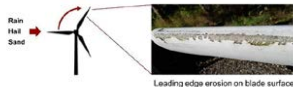
Figure 1: The leading-edge erosion phenomenon on the wind turbine blade surface.
