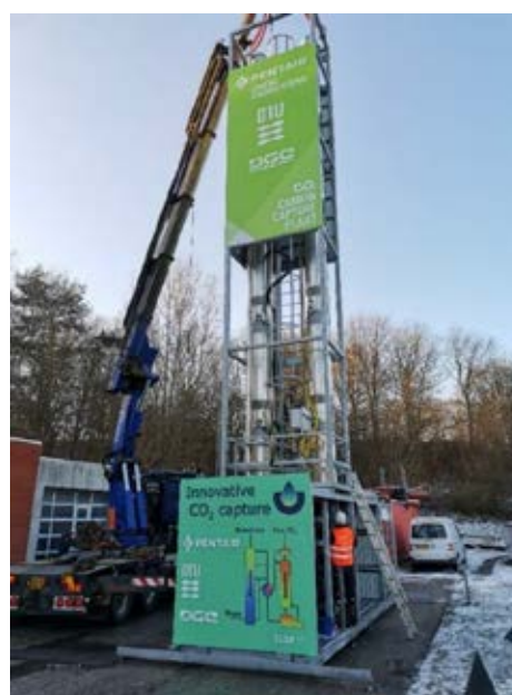
Figure 1: The newly constructed mobile test unit for biogas upgrading raised at Mølleåværket A/S.
