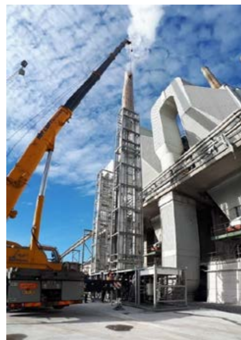
Figure 1: The mobile capture plant being commissioned at Aalborg Portland.
