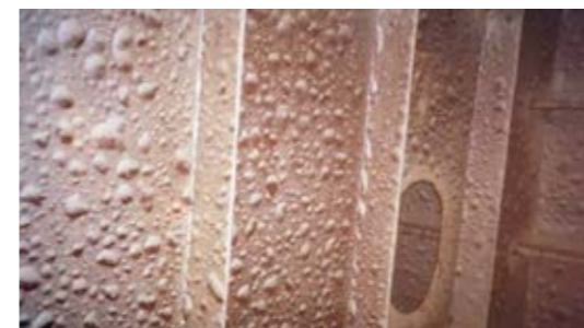
Figure 2: Coated steel surface exhibiting a blistering defect [6].
