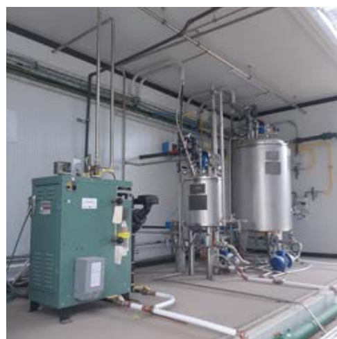
Pilot installations for the biosuccinic acid production from sugar containing side streams [1]. Enrique López de los Mozos
