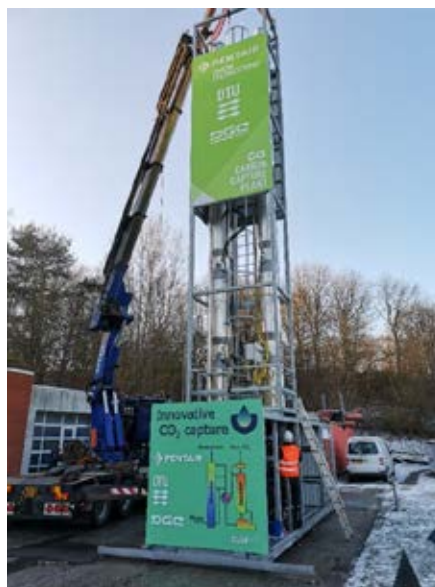
Figure 1: The newly constructed mobile test unit for biogas upgrading raised at Mølleåværket A/S.
