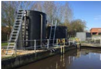
Figure 1: MABR reactors at the Ejby Mølle WRRF in Odense, Denmark.
